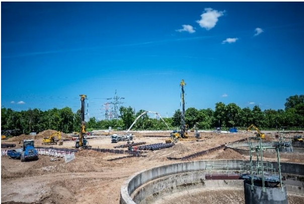
(4) Drone footage documented the progress of construction and the total volume of excavated soil, which amounted to 45,000 m 3 .
