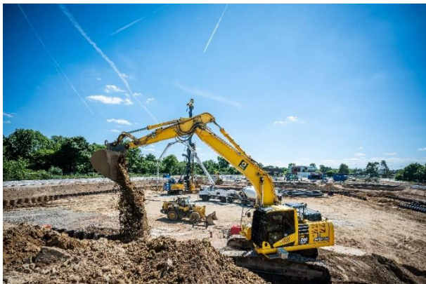
(1) Precision in action: The Semi-GPS 3D excavator grades the subgrade with an accuracy of up to 2 cm.
