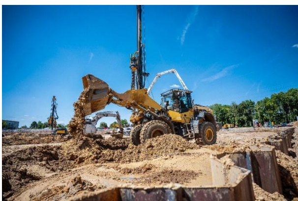
(2) A strong partnership: Bauer Resources and Bauer Spezialtiefbau worked hand in hand to complete the excavation on schedule and to exact specifications.
