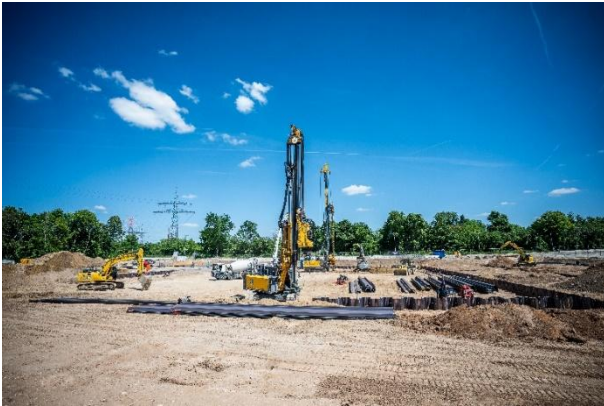
(3) U-Jagged sheet pile panels were precisely inserted using an RG 19 T. The piling work was carried out using a BG 30.
